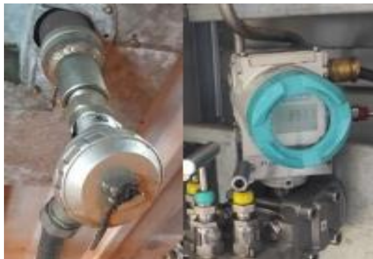
(a) (b) Gambar 3. Alat ukur: (a) Temperature Transmitter, (b) Pressure Transmitter
